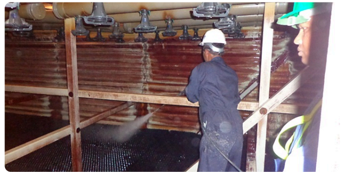
Nozzle inspection and replacement
